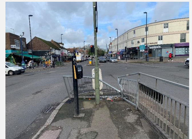
Damaged guard rail
