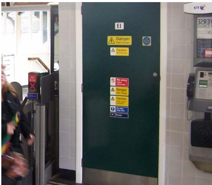
Figure 3.1: Electrical equipment room 1/661
