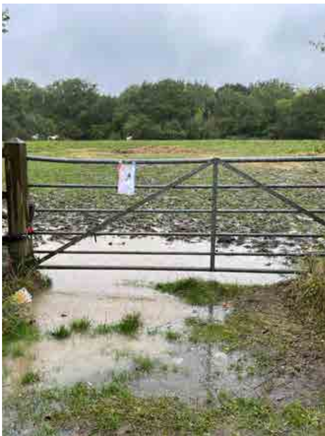
Surface water flooding at appeal site access
