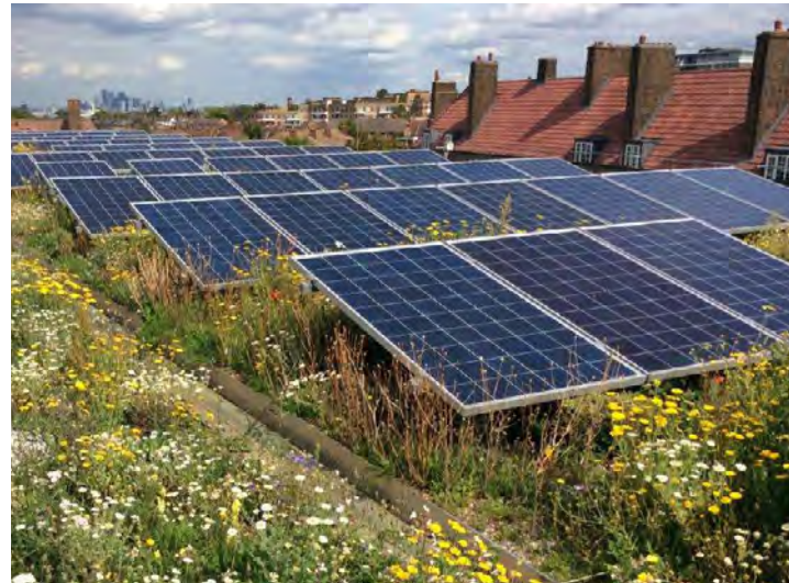
Figure 4.12: Photovoltaic panels on the roof
